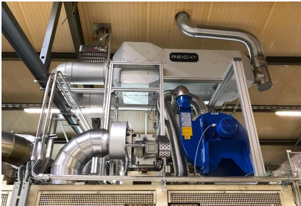
Printing Industry - Panel Sheet Printing Capacity: 350 Nm 3 /h
